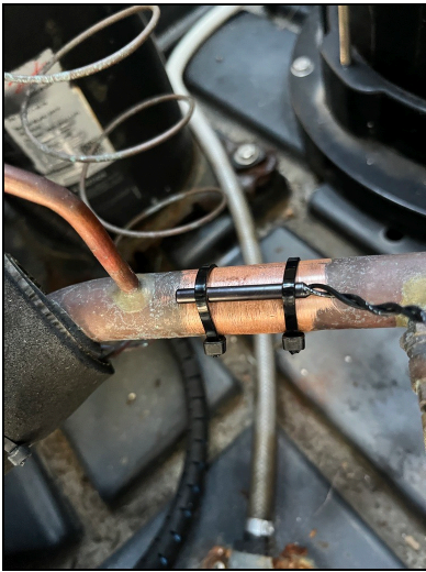
Figure 4 - Sensor on Suction Line
