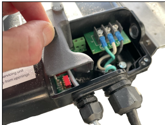
Figure 6 - Inner Wire Cover Removed
